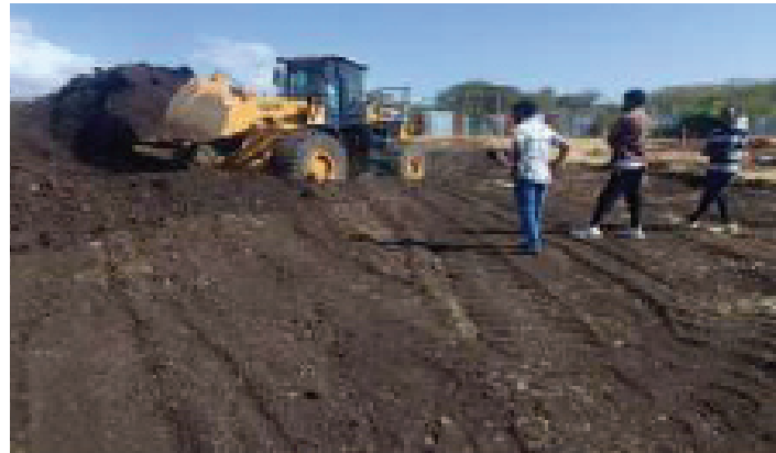
Arbaminch elders Center
